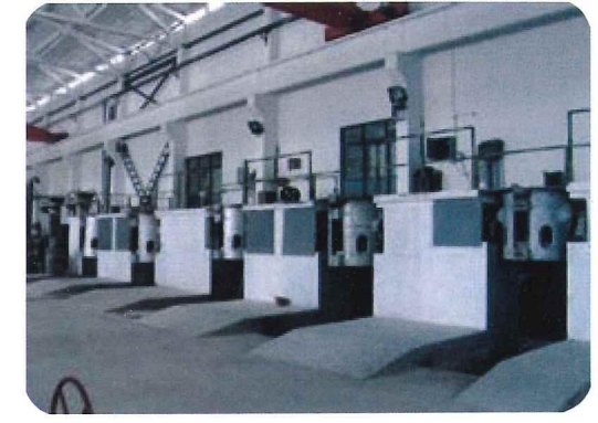
© Non-vacuum smelting casting equipment, Function: Smelt and cast high-temperature alloy, stainless steel, carbon steel, aluminum and other casting. 500kg intermediate frequency fumaces, 1 set; 300kg intermediate frequency fumaces, 1 set; 150kg intermediate frequency fumaces, 2 set;
